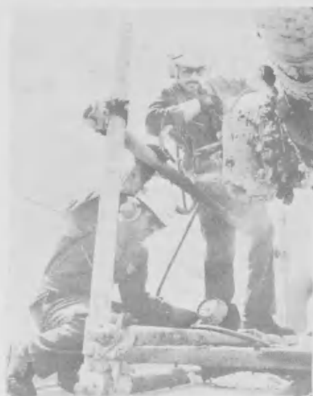
Furmanite technicians here inject a special sealing compound into holes previously drilled and tapped # 2 Powerhouse.
